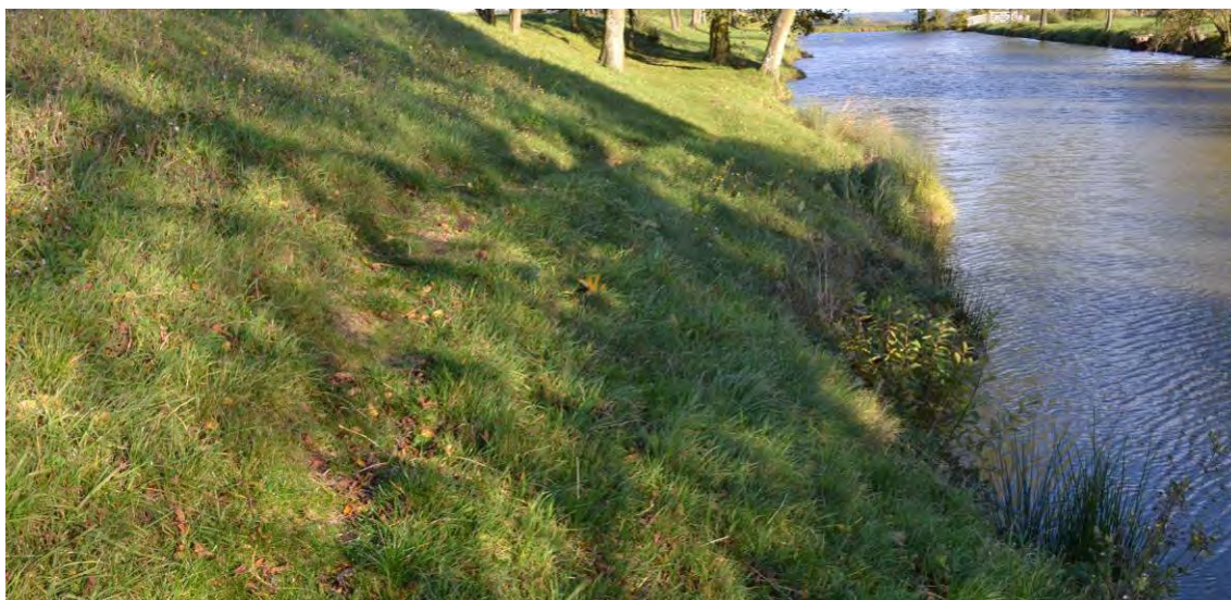
Fig. 5/27 Erosion and slumping at the base of the West Pyramid Mount, and damaging desire-line path
